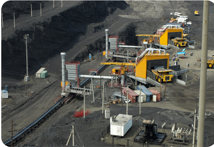
Fig. 1. Commissioning of a cyclic flow stripping complex (CPVC) at the Vostochny section
